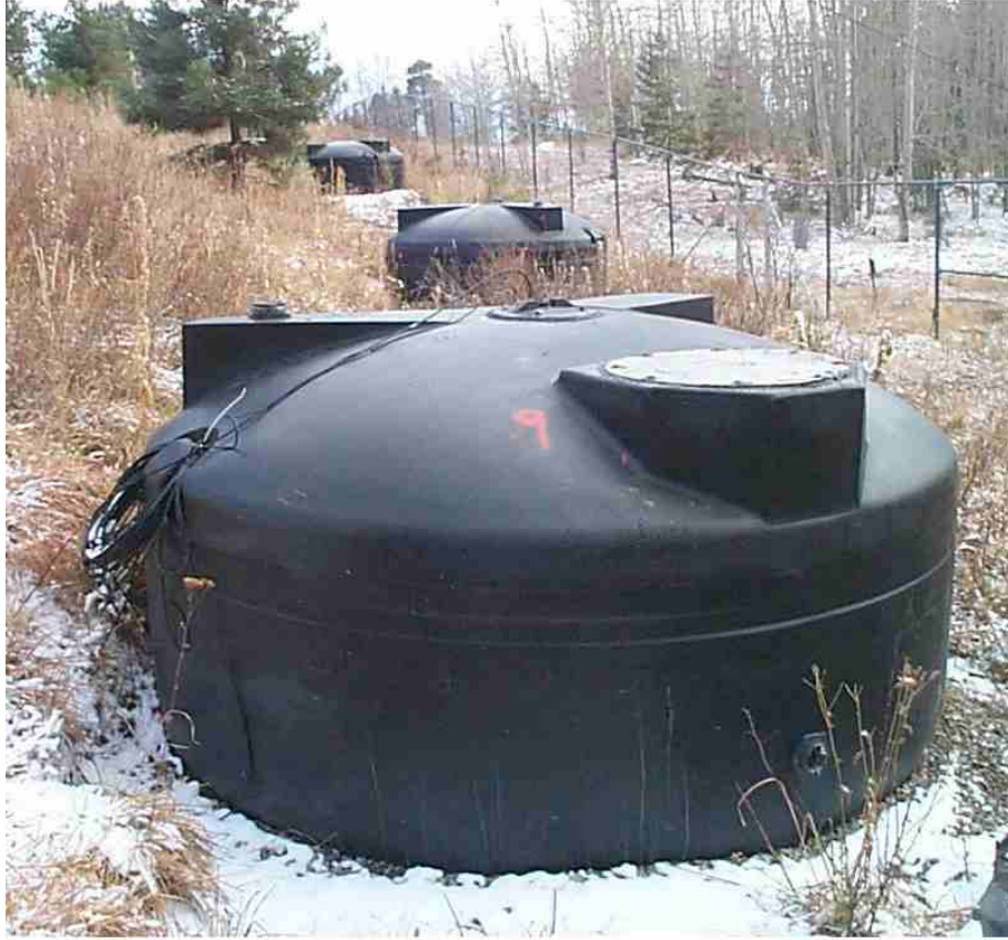
Figure 5.7: Photo of an outrigger tank.
