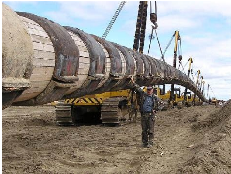
Building typical ground pipeline. Requires ground right of way and results in damage to ecology
