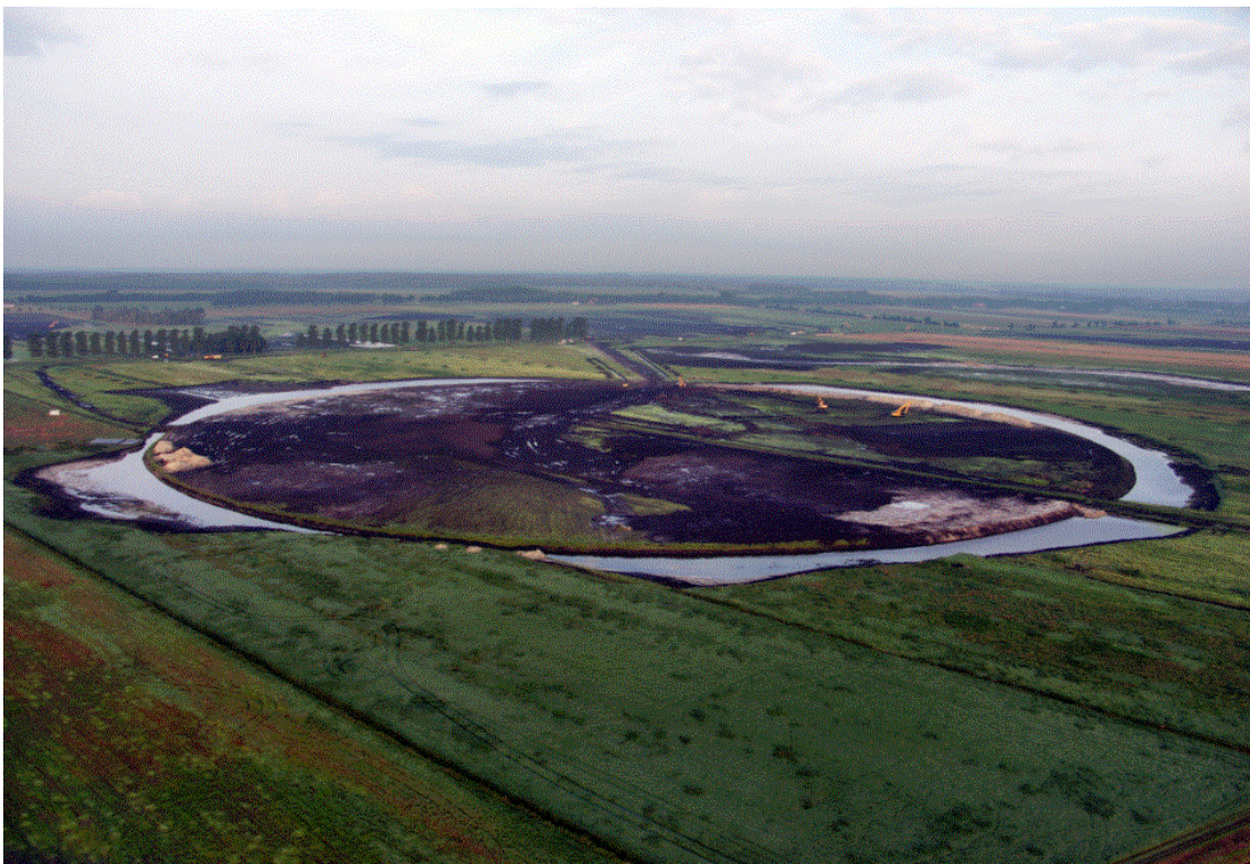
Figure 1: the LOFAR “super-terp” under construction and as it appeared around the time of the EVN IX Symposium (September 2008). The “super-terp” is raised ~ 1 metre above the local ground level and measures 360 metres across. Six of the thirteen LOFAR core stations will be located here. The other 7 core stations are located within a few km of the super-terp.
