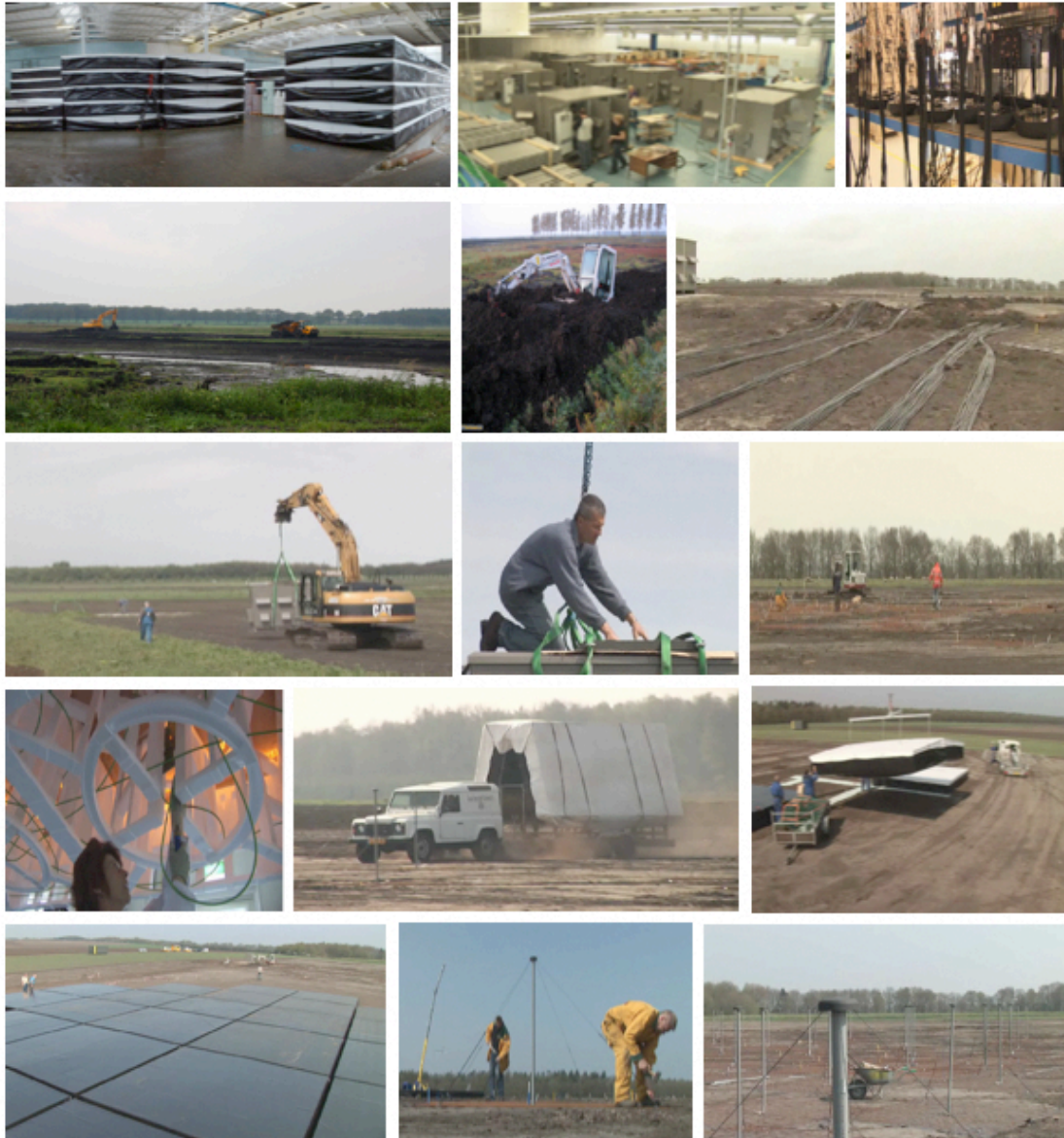
Figure 4: Some of the stages involved in building LOFAR – producing and storing the antenna hardware, preparing the fields, placing the cabinets, digging in the cables and finally deploying the HBA and LBA antennas.
