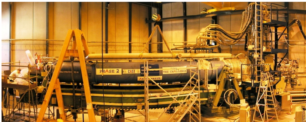
Figure 2.14: A picture taken during the installation of the expansion volume on top of the CAST magnet.
