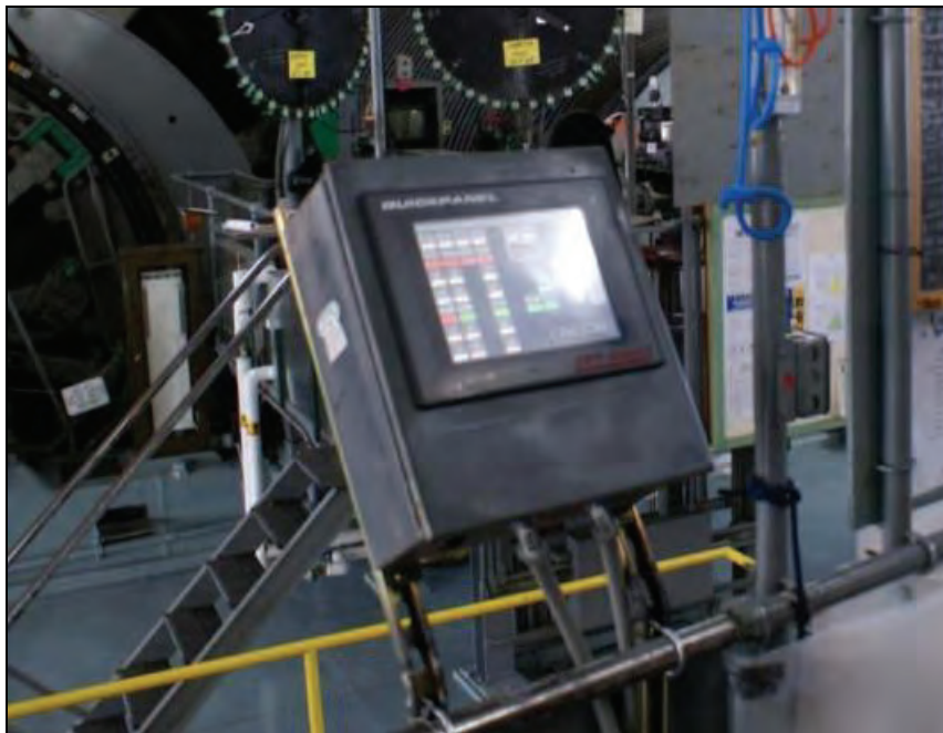
Figure 5.5.2-3 Existing QuickPanel operator Interface at a hoist operator work station.
