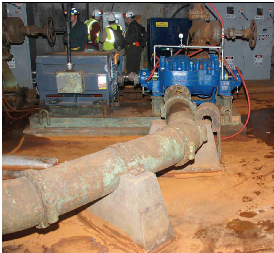
Figure 5.4.3.11.3 Pump station at the 3650L. [SDSTA]
