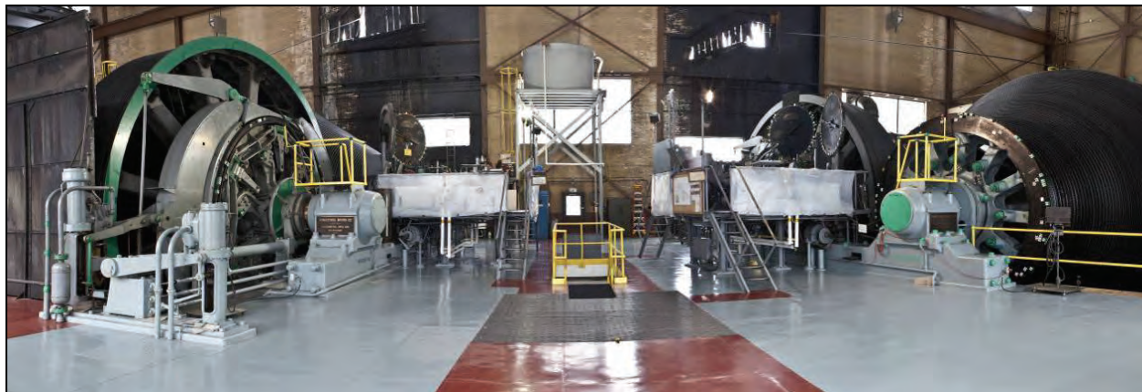
Figure 5.4.3.2.1-2 Ross Hoists. [Matt Kapust, DUSEL]
