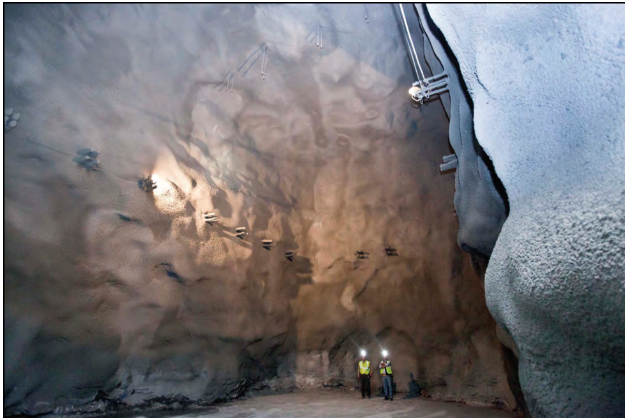
Figure 5.6.7-2 Inside the DLM excavation facing south after shotcrete application; DLM dimensions are: length 60 ft (18 m) x width 30 ft (9 m) x height 50 ft (15 m). [Bill Harlan, DUSEL]
