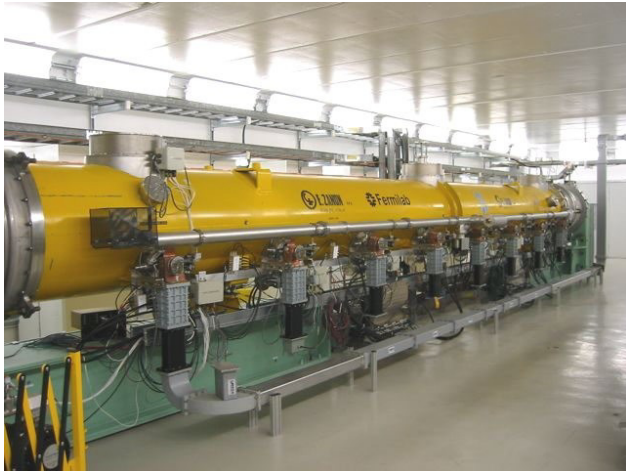
Figure 2: First installed Cryomodule (CM1)
