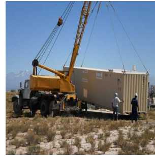
Figure 8: The new shelter for the upgraded CLF is placed in position at the site.
