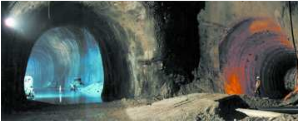
Figure 8. Excavations for National Laboratories of Gran Sasso. Deep underground experiments at sites like this are shielded by the earth above from most background effects, and are complementary to accelerator experiments at laboratories like the LHC. Credit: INFN
