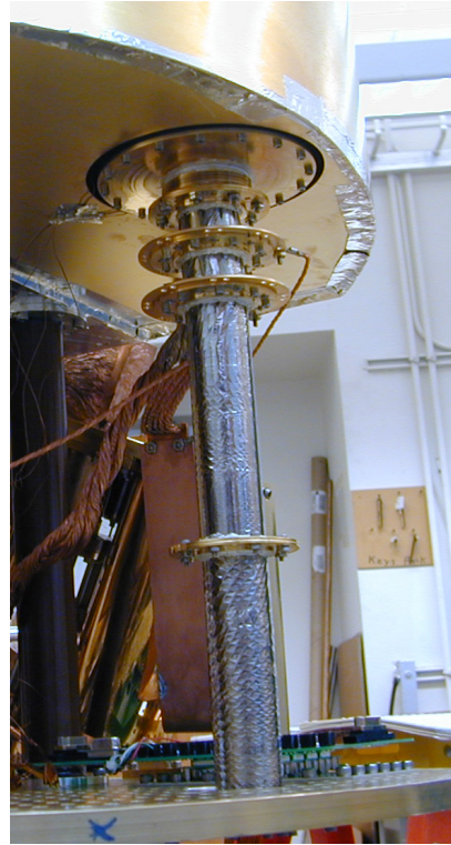
(b) RF tower assembly in situ.
