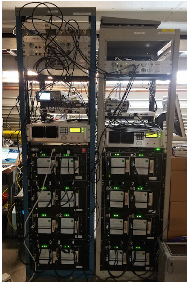
Figure 6. VLBI backend installed at the SPT control room. These racks comprise a 64Gbps data recording system.
