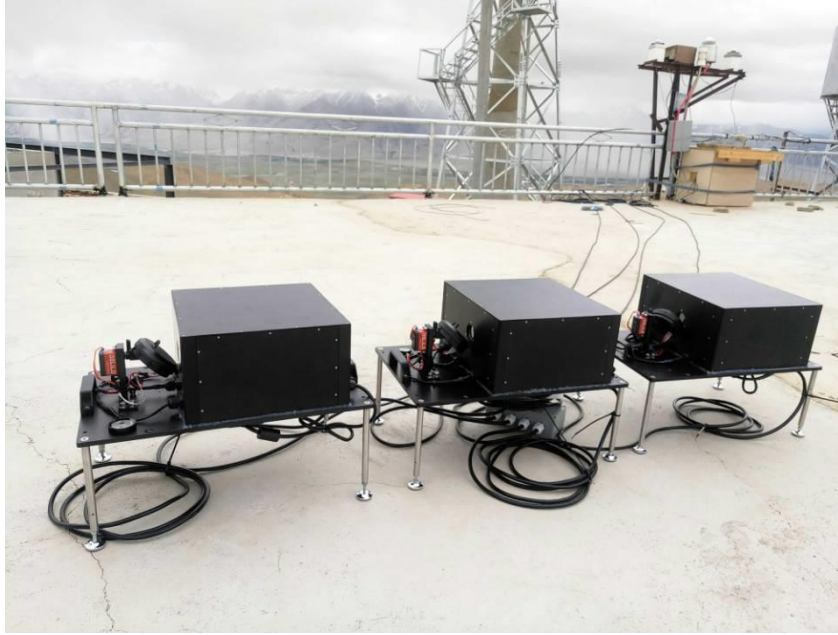
Fig. 16. NISBM installed at Nagri Observatory
