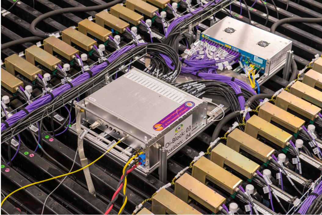
Figure 7: Photograph of a power distribution box (foreground) and data concentrator module (background) on top of the far detector. Black 6-conductor power cables run from the power distribution box to the front-end boards (copper). Violet CAT5e cables run from the data concentrator module to the front-end boards. The ground braid, sense cable (gray), high voltage cable (yellow), 3.5 V cable, and 24 V cable can be seen connected to the back of the power distribution box. The front-end boards and APDs are inside the copper enclosures.
