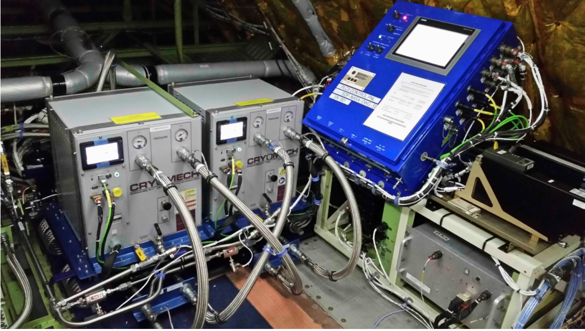
Fig. 15. Compressors located on the upper deck of the SOFIA Boeing 747.
