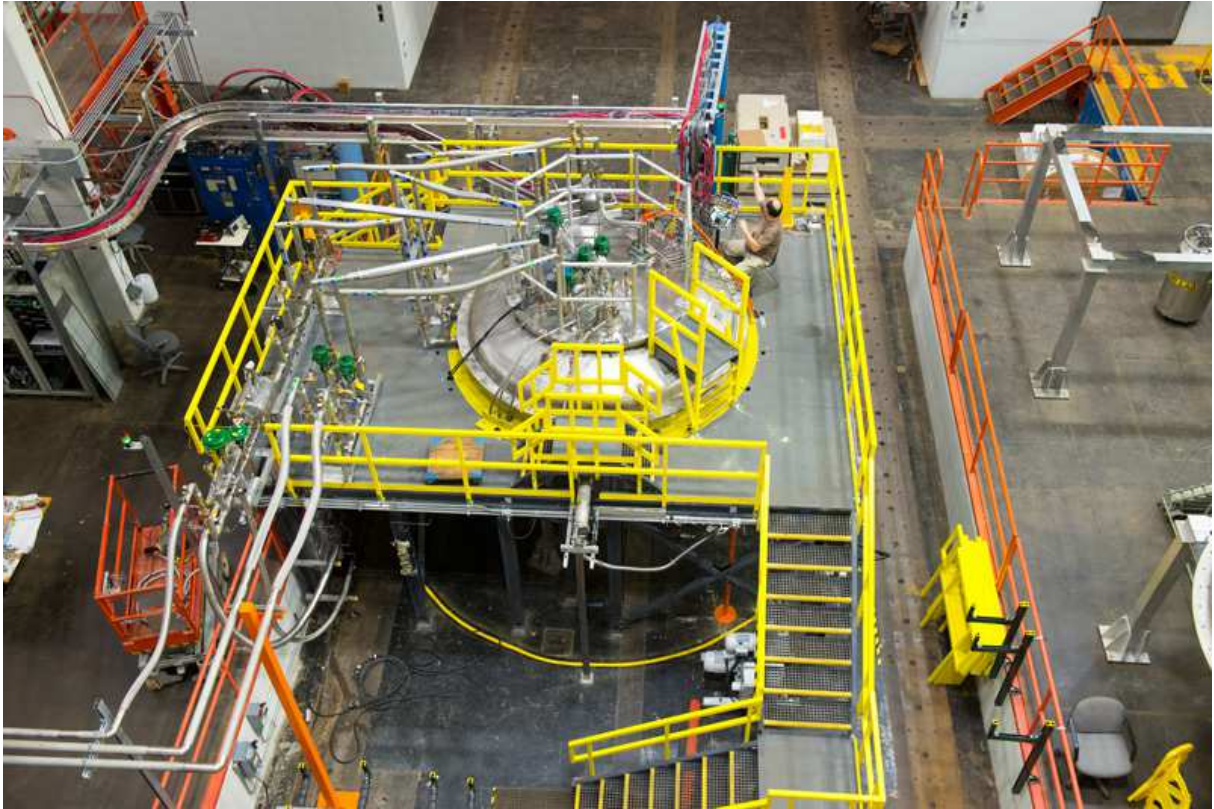
Figure 2. Photograph of the existing installation of the vacuum vessel, including the associated work platform and cryogenic infrastructure. The vacuum vessel was formally used as a liquid helium test stand for solenoids for the Mu2e project. Picture credit: Fermilab
