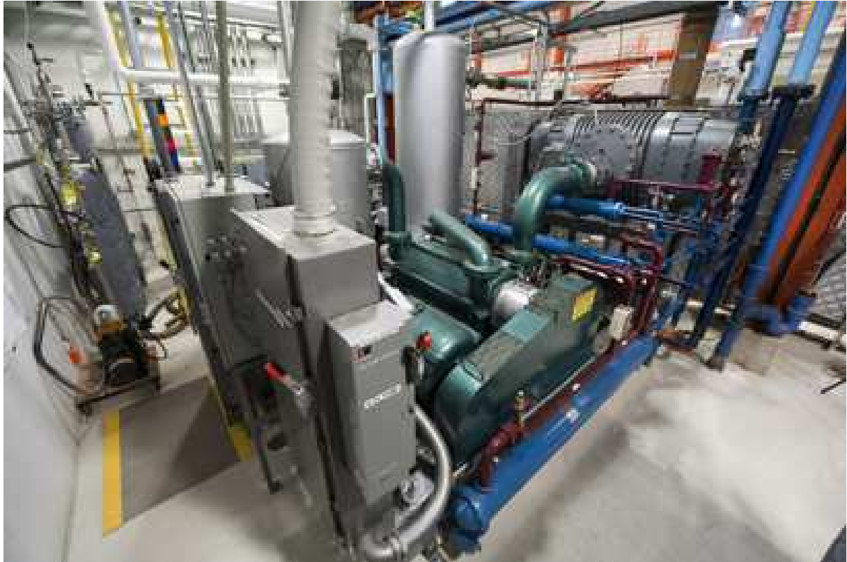
Figure 5. Example of a pumping system for the superfluid helium system, consisting of a Kinney vacuum booster and liquid ring pump.
