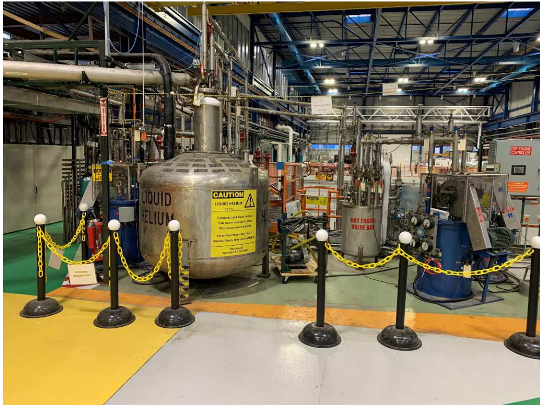
Figure 3. Photograph of the helium cryoplant, including the 2000 liter liquid helium dewar on the left. The plant is rated at a refrigeration capacity of 625 W at 4.5 K or 4.2 g/s of liquid helium.
