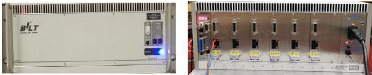
Figure 18: Steerers power supplies main-frame front (left) and back (right) equipped with several PSs modules.
