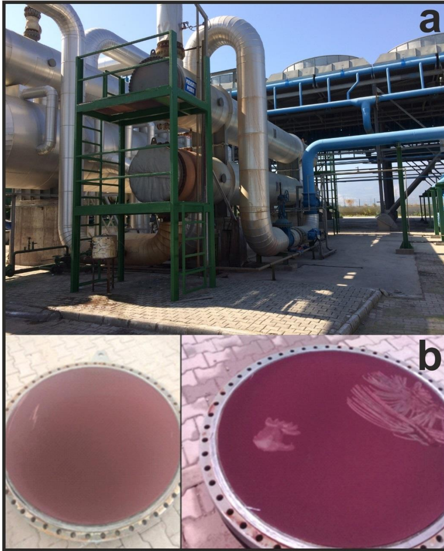
Figure 16. Sb scale encountered in the preheater in the ORC-binary system in the GGF a) Preheater in, b) Sb scale in the preheater system (Photo credit: Beştepelers company)
