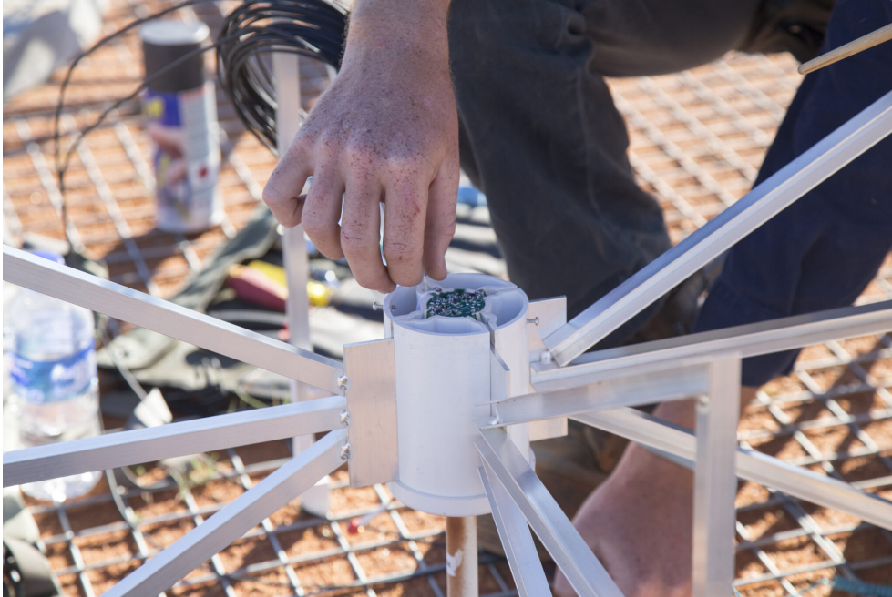
Figure 2.5: Low-noise amplifier (LNA) of the MWA is attached to the bowtie dipoles (Image credit: ICRAR/Curtin).
