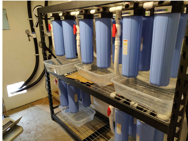
Figure 7: The interior of the water hut showing the filtration plant.
