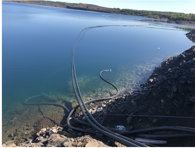
Figure 8: The completed inflow and outflow water pipes for the detector. The third, shorter pipe is the water intake from the mine pit, which was used for filling the detector during deployment.
