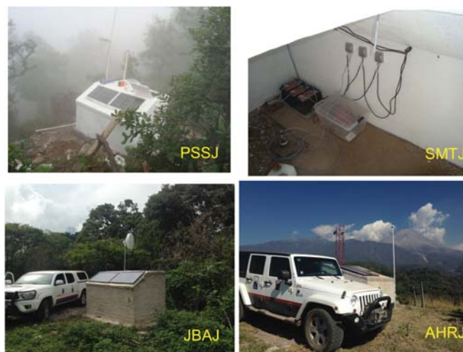
▲ Figure 5. Seismic stations sheds for housing equipment at each site.
