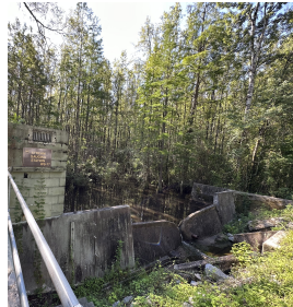
(h) Flow measurement station
