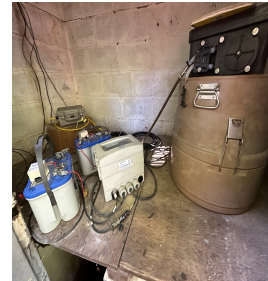
(i) Recording logger in a gauge house
