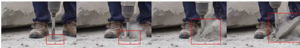
(b) Caption: A worker uses a pneumatic chisel to break apart a large chunk of concrete, sending debris flying. Human-judged Physical Violations: A large piece of concrete cannot spontaneously form from the dust and debris generated by the drill ( Conservation of Mass, Material Properties ).
