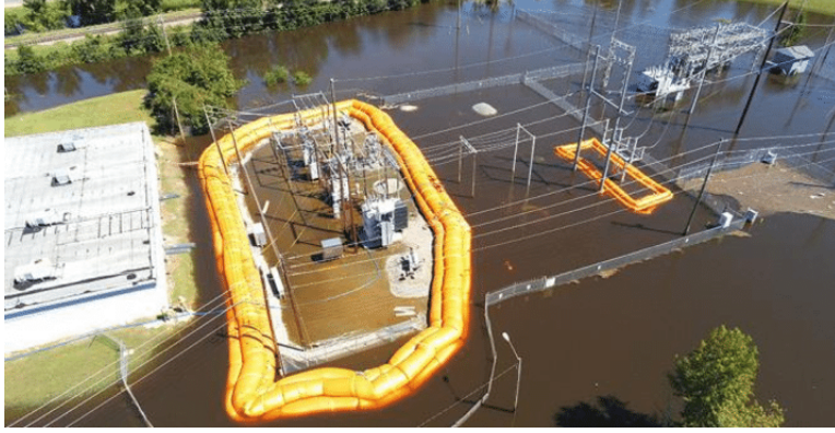
Figure 1: Tiger Dam protecting a substation in North Carolina after Hurricane Florence
