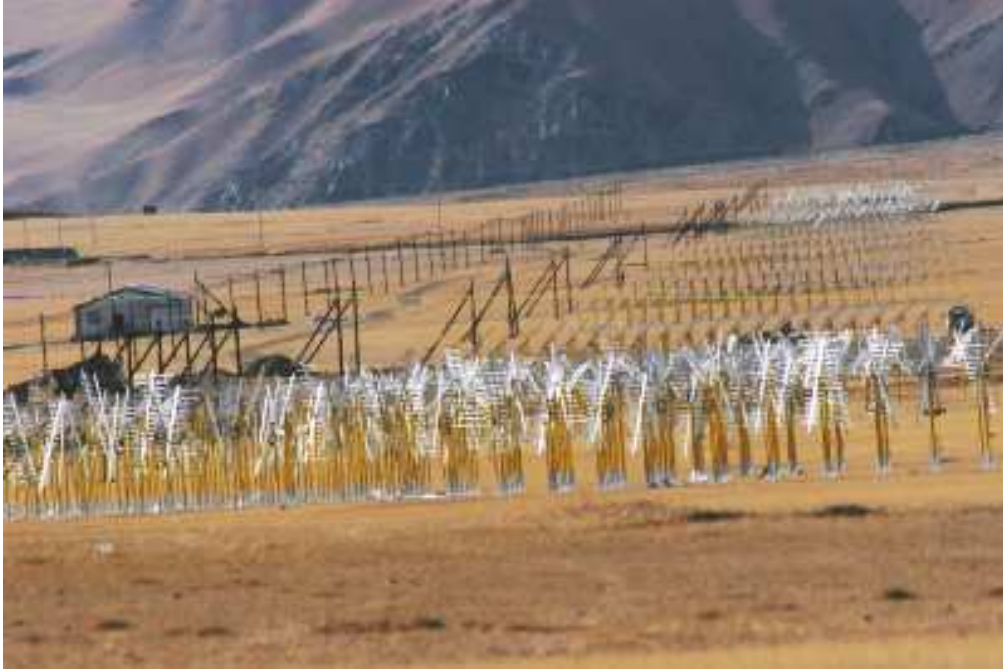
Figure 5. Status of PaST, December 2004. Over 2000 antennas have been installed and about half of these have been aligned at the North Celestial Pole. A 170 square meter building has been constructed. Power mains supply the site, as do copper telephone and internet connections. A 3 km optical fiber trunk to carry signals from the phased arrays is in place.
